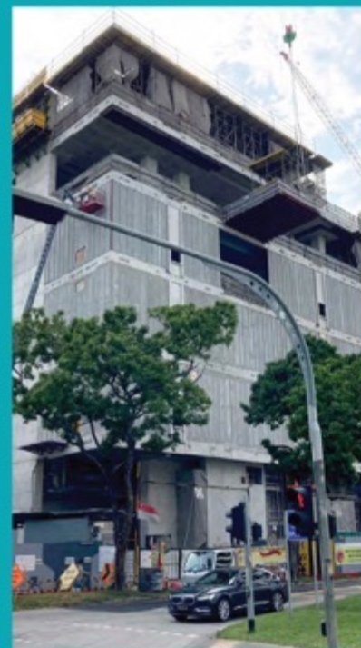
STTelemedia Global Data Centres at S1 Defu Lane 10
